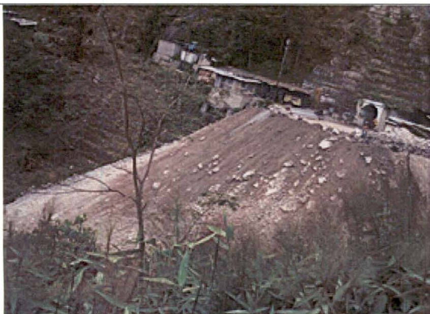
Photograph 8.5 Dumping of Tunnel wastes along the hill slope near Linsebong, Rammam project invite site for future landslide.
