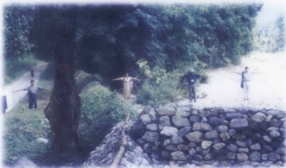
Photo. 6.2 Embankment induced river bed rising at the Bala valley near Santalabari.
