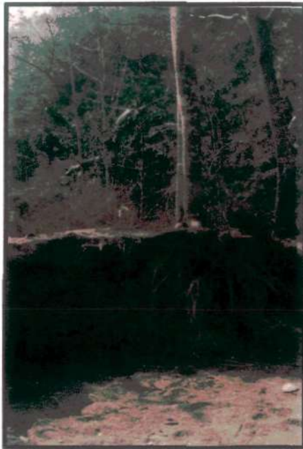
Photo 5.2 Bank erosion - rampant in the Southern piedmont zone
